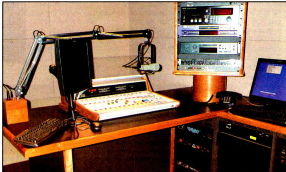
Cumulus expanded the available counter space by asking to have the announcer panels mounted in the mic risers.
