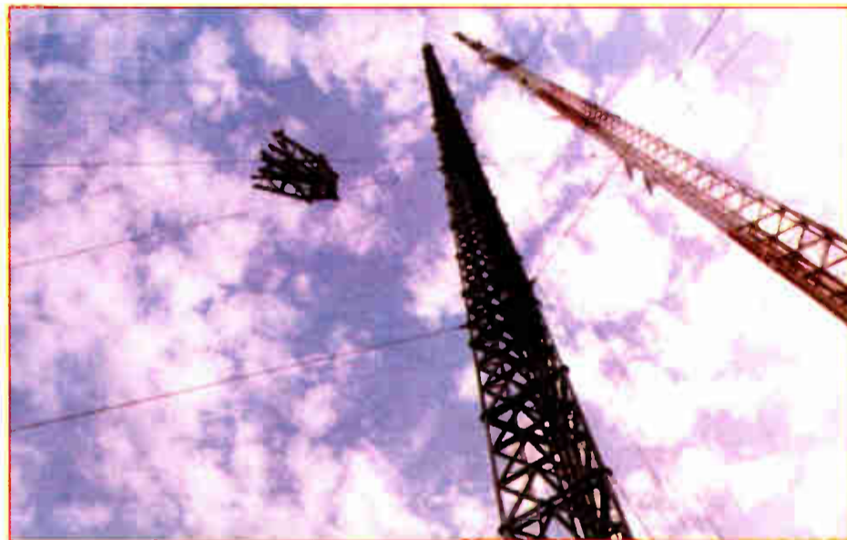
The 'arbor' is lifted into place for a candelabra-type tower being constructed next to an existing structure in a photo from Dielectric Communications.
