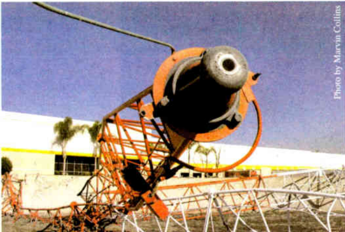
The top half of the base insulator is seen, still attached to the bottom of the fallen tower. The insulator pair supported the 400,000-pound steel KFI tower.
