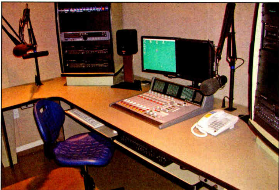
A view of an Edit room. Equipment includes Shure SM7 mics, Omnidax studio furniture, an ESE master clock system, Telos Systems 2101 phone system, Audion Labs VoxPro digital voice editors and Enco DADpro32 digital automation.
