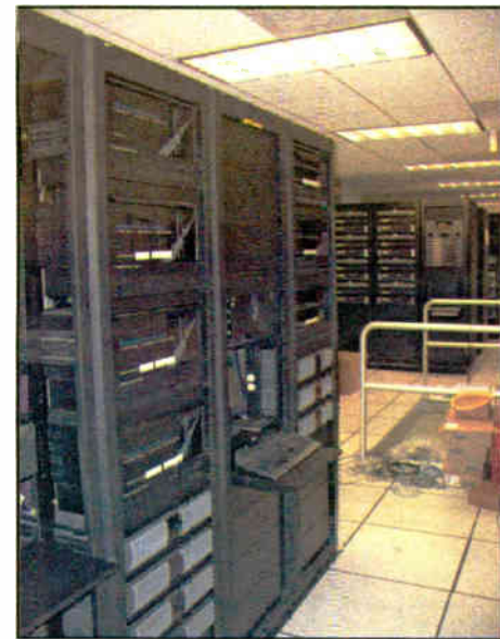
Server room, including Bridge Routers.
