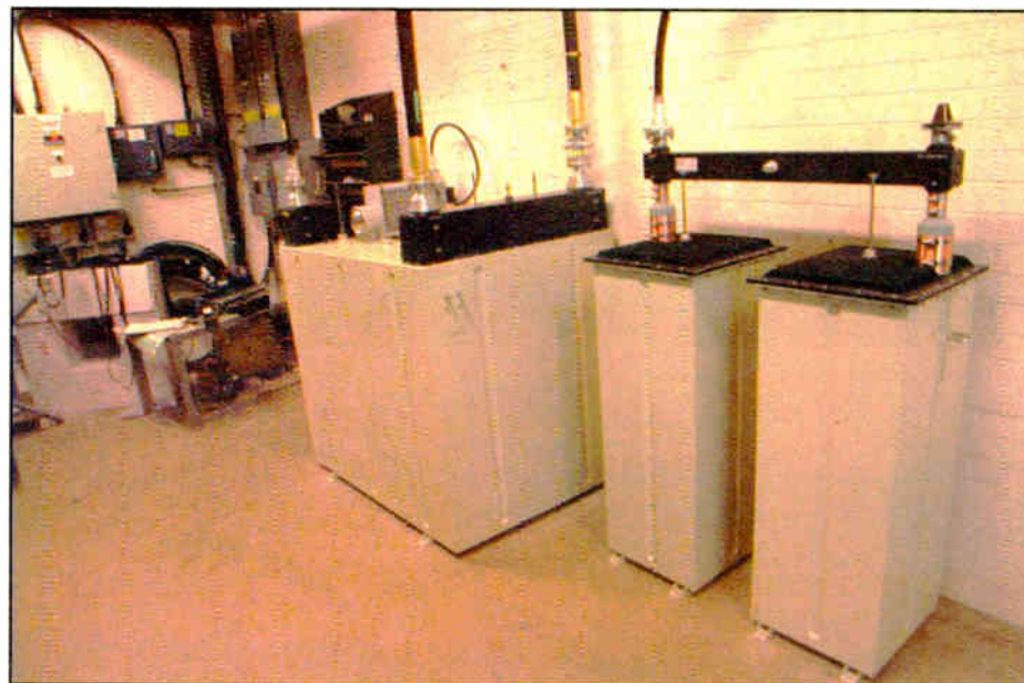
RFS's custom combiner achieves 500 kHz channel spacing for the Kerrang! FM service at Crown Castle's Sutton Coldfield site in the West Midlands.
