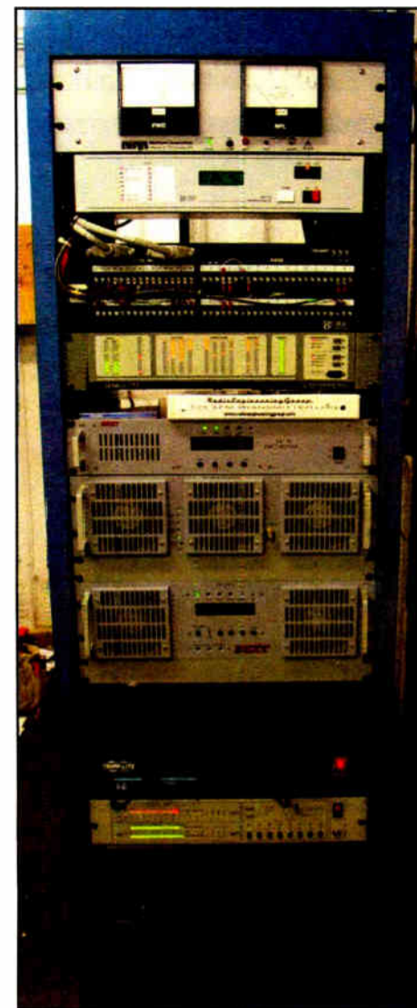
KCEE(FM)'s transmitter rack.
