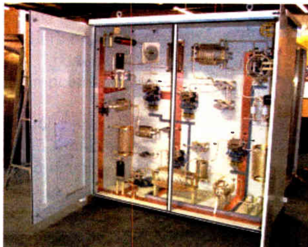
DIRECTIONAL ARRAY ANTENNA TUNING UNIT GAITHERSBURG, MD
