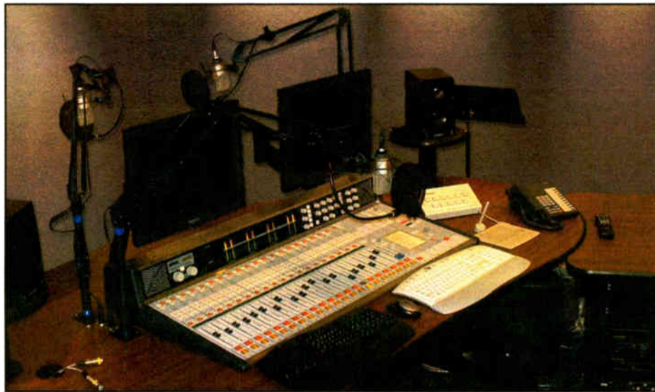
Creative Studio Solutions designed the new production room for KKPT(FM), which uses a Wheatstone D-8000.
