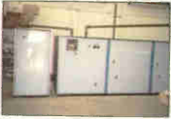
DA Phasing System Cabinet KMJ Radio Fresno, CA 4-Tower 50kW 580KHz
