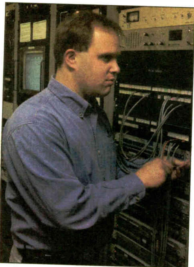
Engineer Mark Wittkoski keeps public radio stations WGUV(AM-FM) and WGV(AM-FM) on the air to keep west Michigan listeners tuning in.
