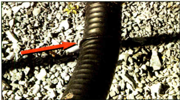
Fig. 1: This transmission line was not supported properly. The crinkle is the result.
