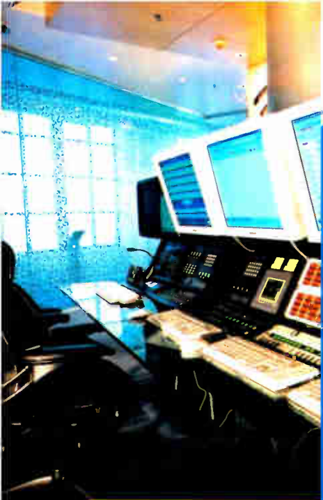
Monitor area of Encoda automation system
