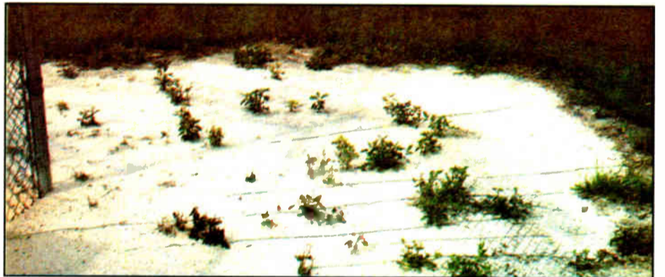
Fig. 3: Exposed ground radials invite a citation
