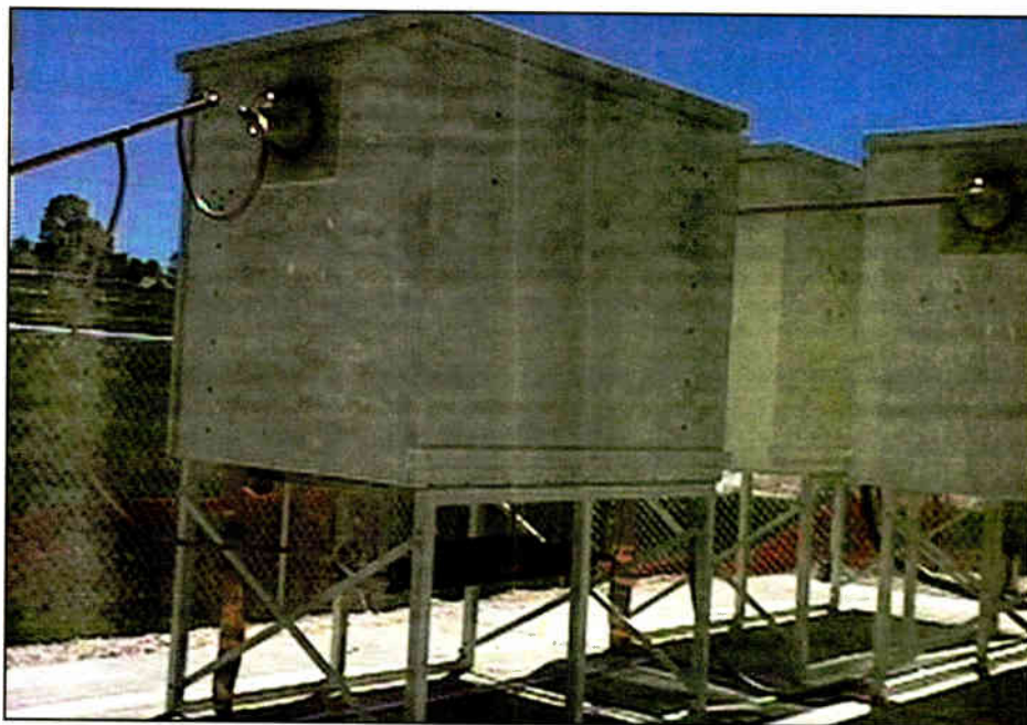
A 30 kW diplexer at AM stations KCMN-KCBR in Colorado Springs, Colo.
