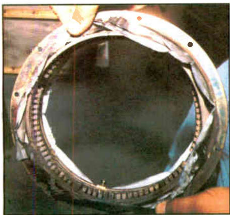
Fig. 1: Inspect tube socket finger stock for broken or bent fingers
