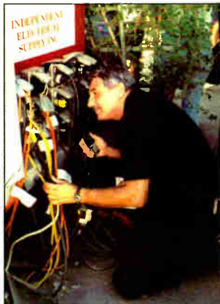
The author is amazed that this power distribution panel works at all
