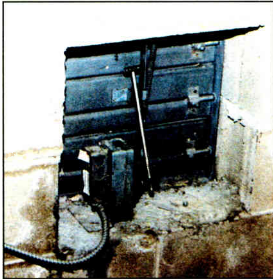
Figure 3: ... and air intake louvers, to provide emergency cooling.
