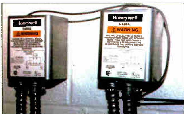
Figure 1: Thermostats monitor the building air.
