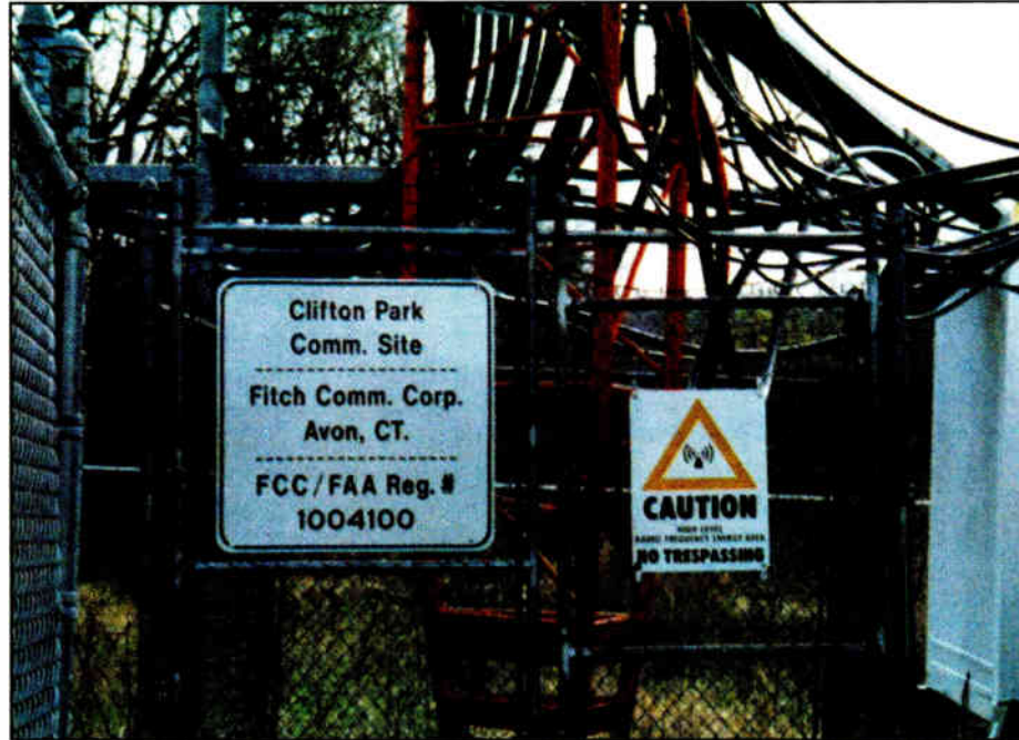
The FCC said of this site, 'The Antenna Structure Registration Number was not displayed in a conspicuous place so that it is readily visible near the base of the antenna structure.'
