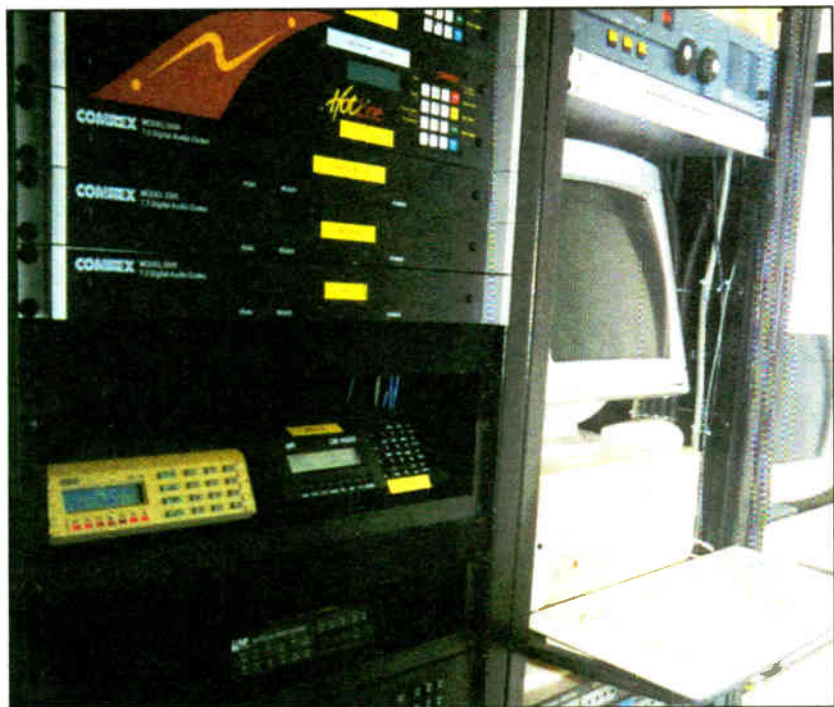
Figure 2: Shown are the completed computer rackmount stand and labeled ISDN gear.
