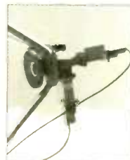
Photo of 7892's mounted between antenna feed and LNA's (both Vertical and Horizontal Polarization).
