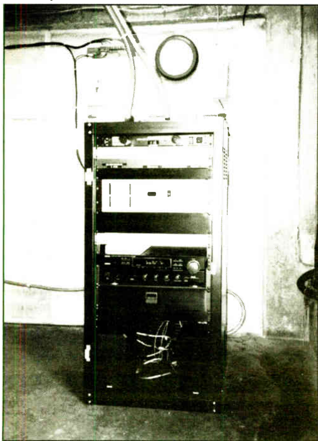
A view of the rack that holds "support" gear
