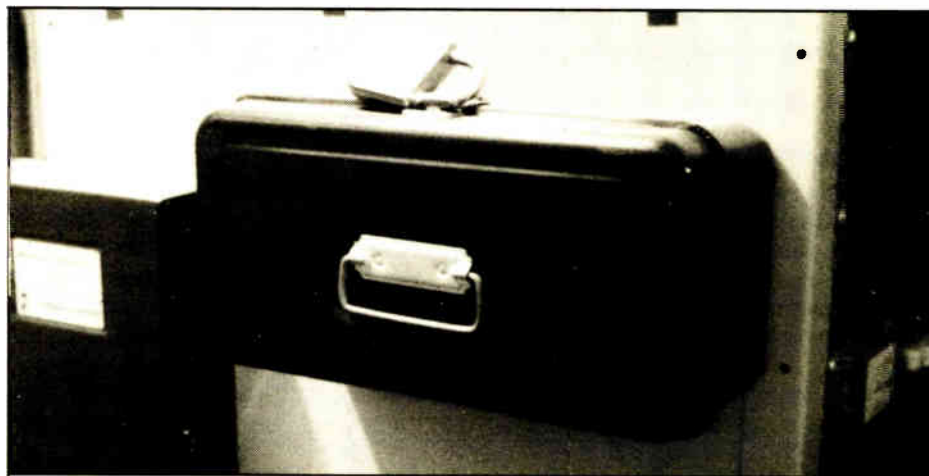
Tools can be safely stashed in a tackle box mounted to the side of an equipment rack in shared transmitter locations.
