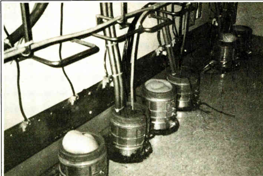
Each studio in KBSG is connected to engineering by two 4" conduits.
