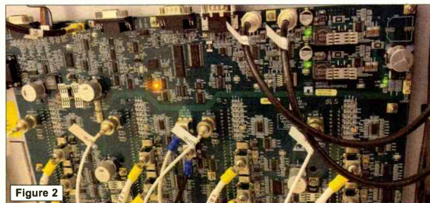
Figure 2 shows a main system PA control board close up, with back door removed. PA backplane connectors can be seen for the four PA modules.
