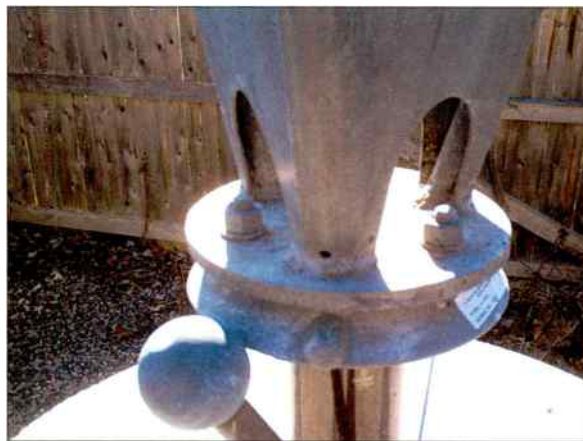
Clear the weep holes on hollow leg towers.
