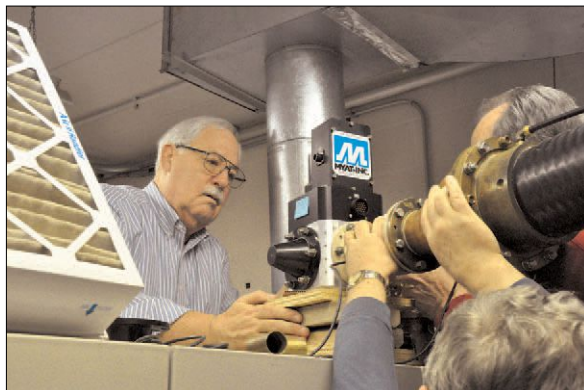
Connecting the 5-inch Coax to the Myat Switch
