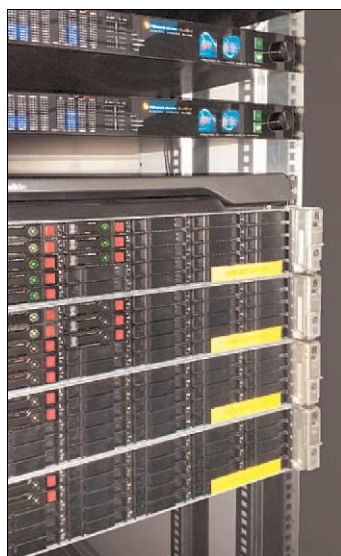
Centralized RCS Zetta automation for four studios running in a virtualized environment with WheatNet-IP audio networking.
