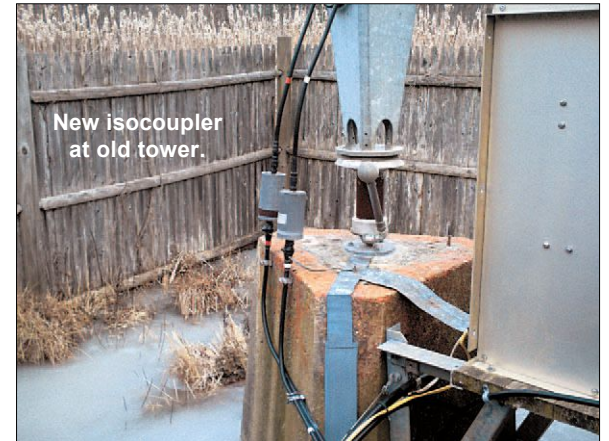
Two isocouplers installed on Tower #1
