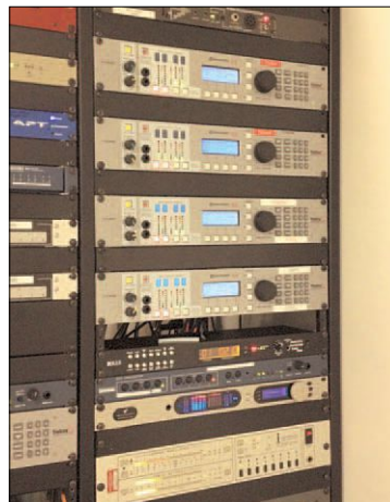
WEKU rack with TieLine Commander G3 units.
