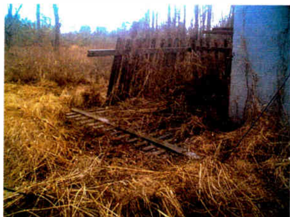
Even before you get to the tower base, you just know there is going to be trouble.
