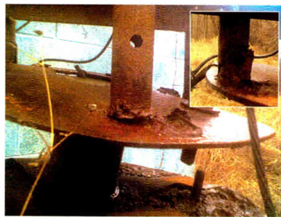
Saying this tower had loose legs was not an understatement.
