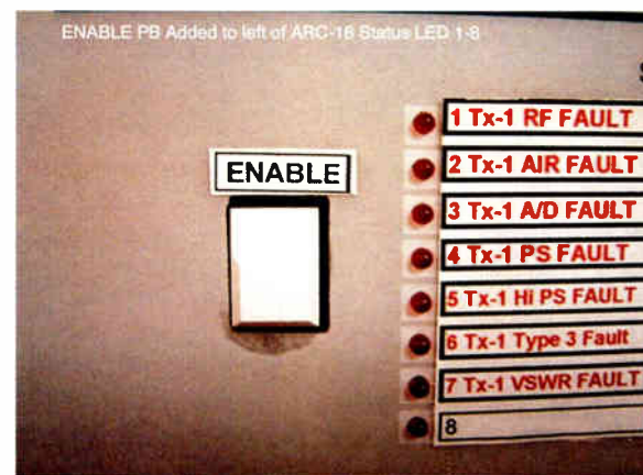
Carefully installed, it almost looks like a factory button.
