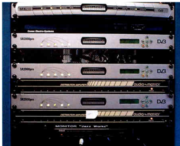
A satellite receiver installation for Content Depot.
