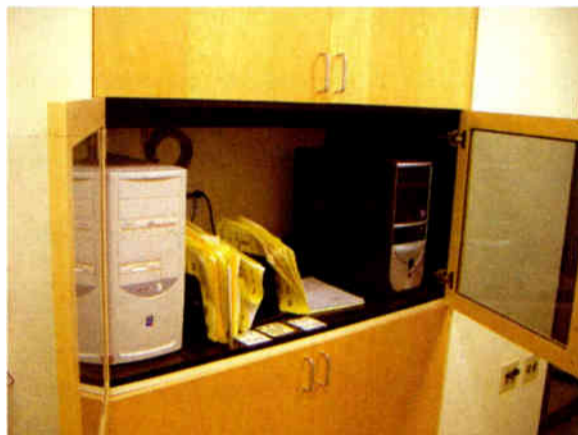
An air conditioned cabinet for the computers.
