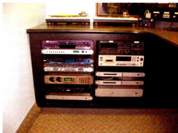
Along with the microphone processors, telephone hybrids and switchers, do not forget the delay unit and accessible "dump" button.
