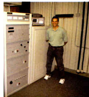
An easy installation and solid operation makes for a pleased engineer.
