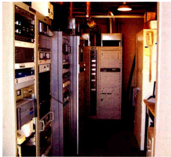
A tightly packed transmitter room.
