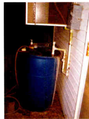
Right from the AC to the storage barrel.
