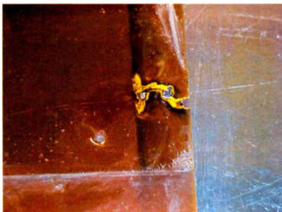
The damage to the blocking cap was obvious.
