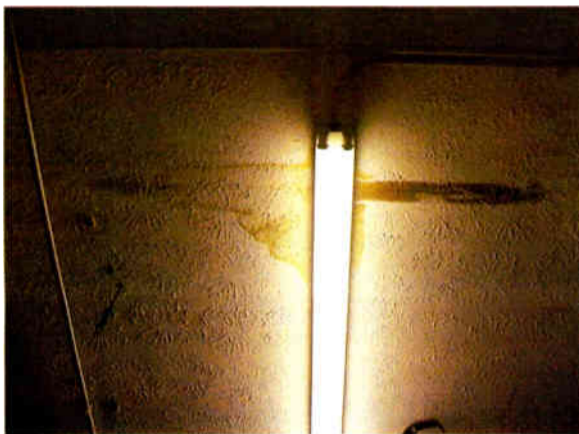
The source of the problem was evident.
