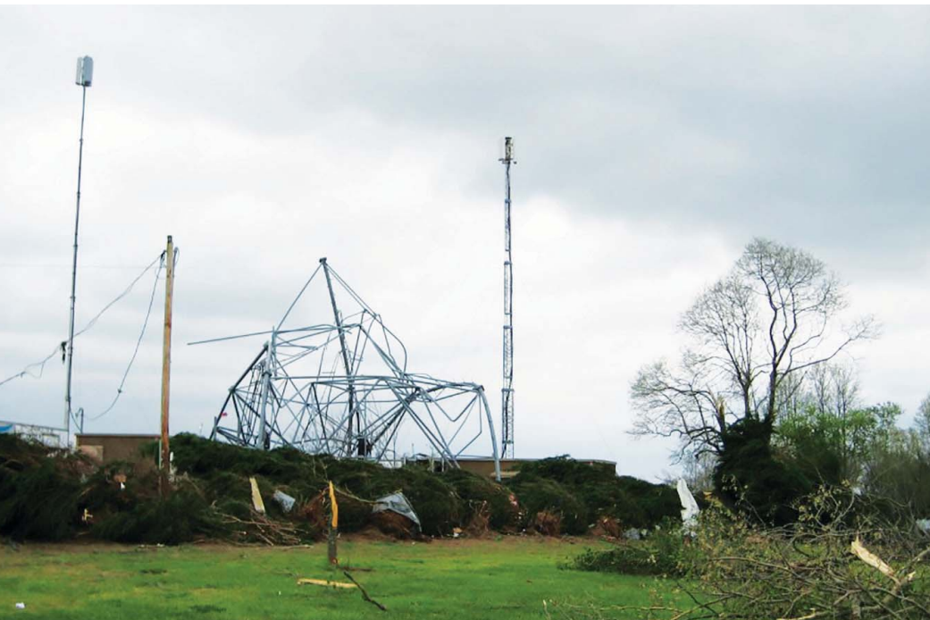
A collapsed cell tower replaced with a portable cellular site with a telescoping mast.
