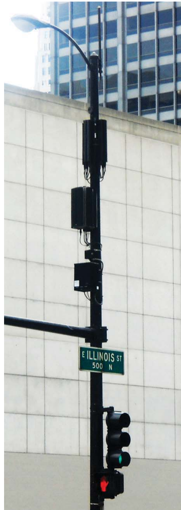
A standard option involves mounting antennas and equipment boxes on a light pole. Photo courtesy of Dewberry
