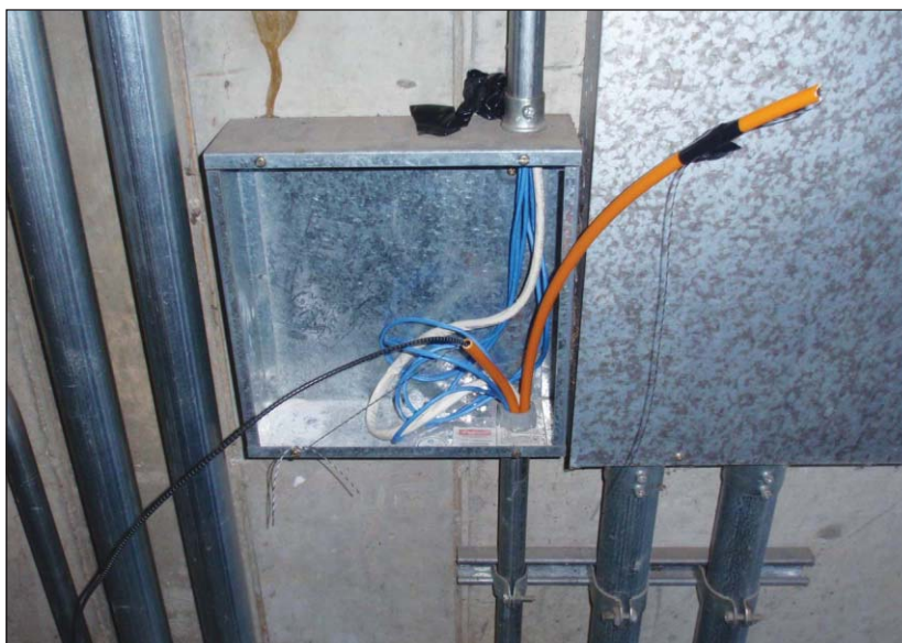
Photo 6. After the microducts were installed from the rooftop to the equipment room, fiber was pulled from the rooftop to the equipment room in one pull through 22 90-degree bends.
