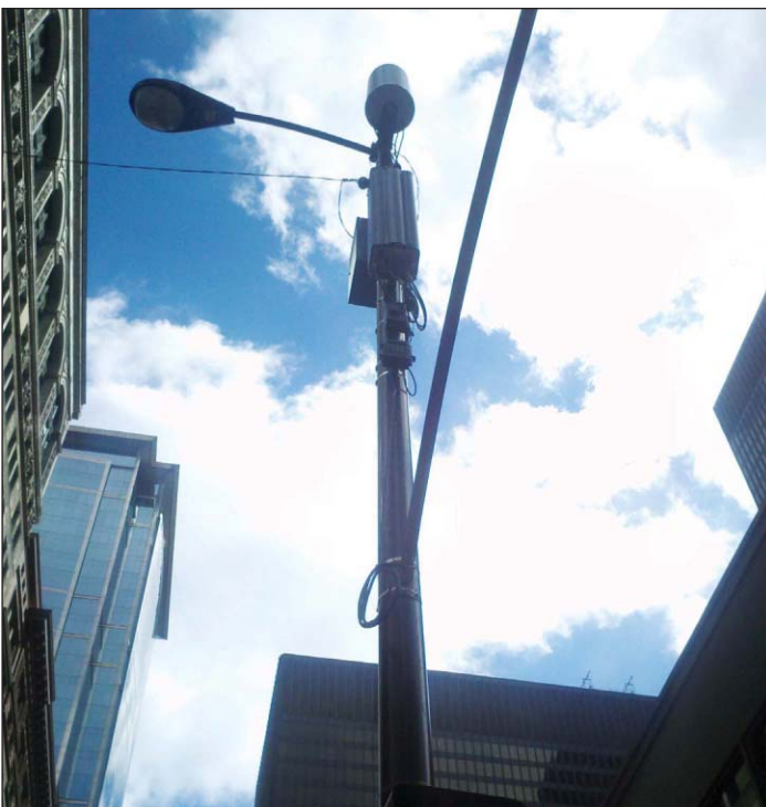
Photo 1. Remote radio heads for distributed antenna systems, such as this node shown on a light pole, often are fed by fiber-optic cable to bring wireless carrier signals to and from the node.
