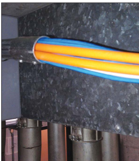
Photo 5. Two 10-millimeter microducts from the rooftop hut to the equipment room were installed, followed by coupling on two microducts that were pushed through the 1.25-inch innerduct to the manhole.
