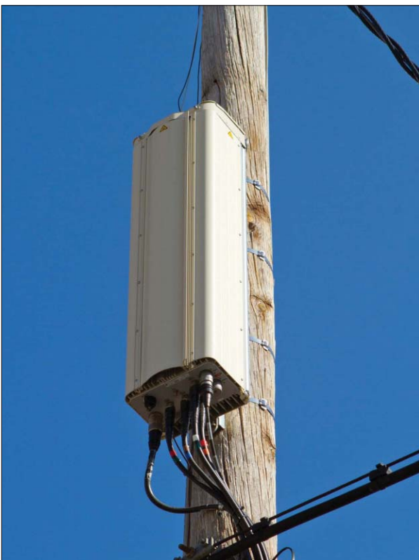
Photo 1. A pole-mounted DAS antenna is connected via a fiber network to the host, which distributes signals from the base transmitter station to multiple remote antenna locations such as this one.
