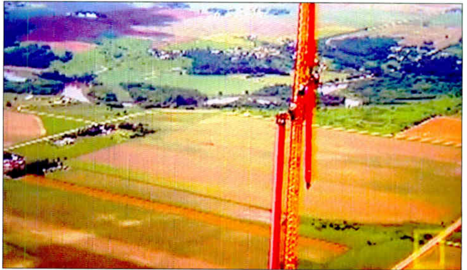
The gin pole lifted the top antenna off of its mounting and the antenna began its descent to the ground, 2,000 feet down.
