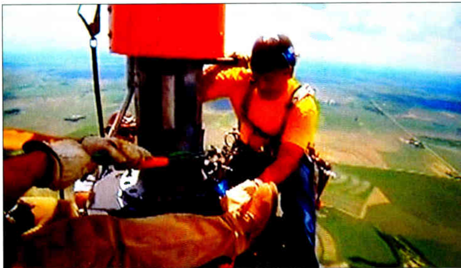
One last bolt on the antenna being removed required leg power applied to the ratchet wrench to dislodge it.
