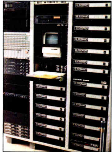
The electronic components are housed in custom racks.
