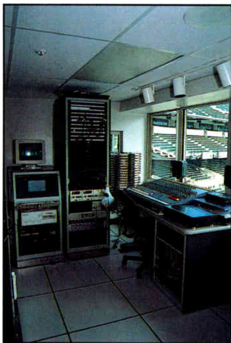
The audio control room.
