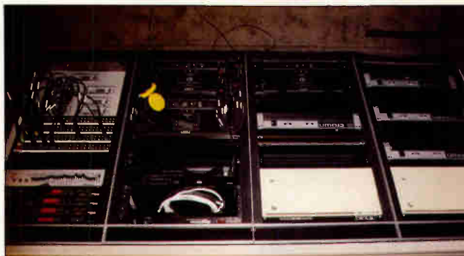
The sanctuary equipment rack.
