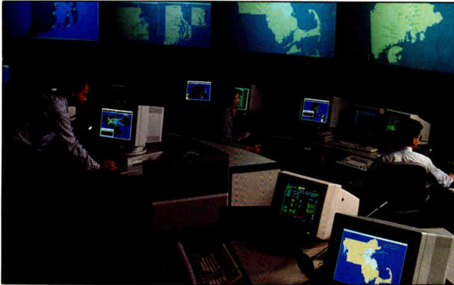
The Crestron media control system and touch screen control serve as the nervous system for N.E. Tel's vast A/V setup.
