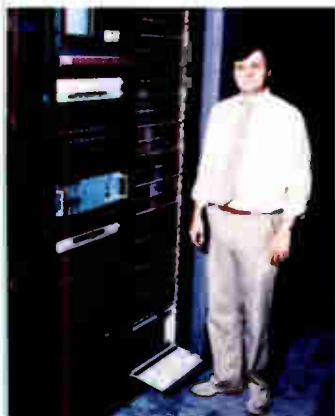
Cibola Systems (Orange, CA) project engineer, Jim Fletcher, installed System 41 at the Los Angeles World Trade Center.
