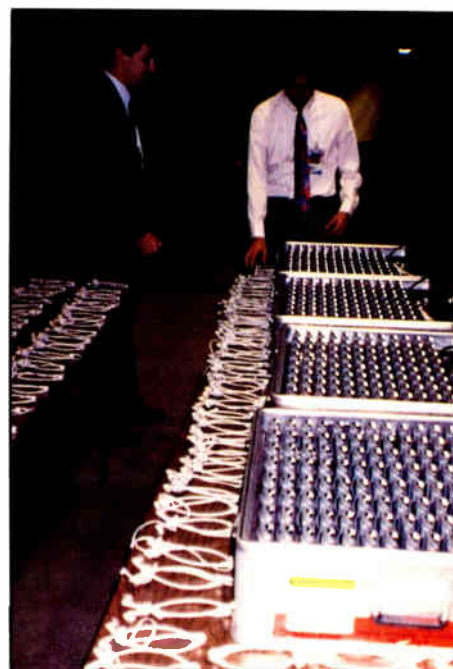
Infrared receivers at the press room of the George R. Brown Convention Center.
