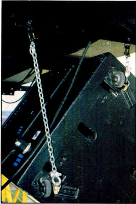
Four chains are used to hang the speakers, but flexibility in the chains and the angle iron allow the cabinets to be aimed in any direction.
