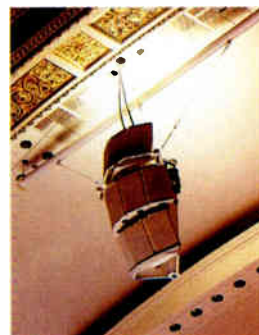
Carnegie Hall A coherent array of UPA-1A loudspeakers, supplemented by MSL-3s and 650-R2 subwoofers (not pictured), is permanently installed for live performance reinforcement..
