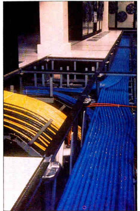
The audio cable travels throughout the building in open trays below raised flooring.
