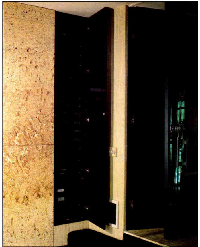
The centralized equipment rack in its own closet in the family room.
