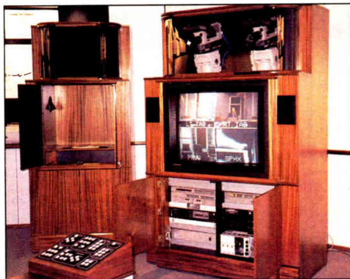
A quad splitter allows previewing of all video signals on the monitor in the teleconferencing console. The graphics console at left can transmit a variety of visual materials (in this case, the x-ray visible in the lower right screen of the monitor).
