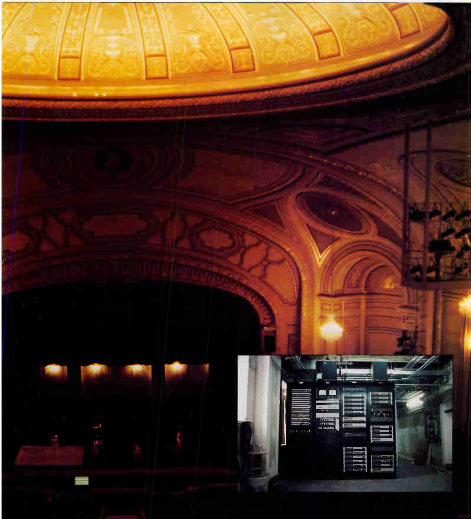
Inset: The house system equipment rack, including CCTV monitors, patch bay, intercom station, and custom control panels.
