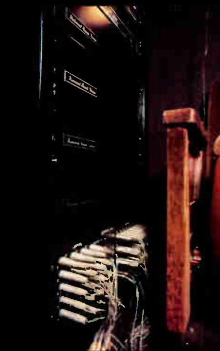
Hookups of the Richmond Sound Command Cue to the theatre sound system is through XLR connectors.
