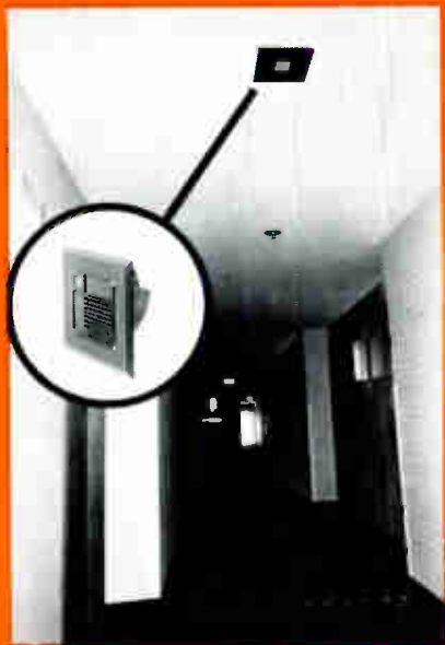
One of the recess-mounted VTF-152U loudspeakers.
