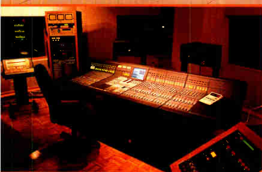
Nashville's Studio III recently completed renovations and installed a 56-input Euphonix CS2000. The studio is also equipped with Otari 24-track analog and Mitsubishi 32-track digital tape machines.
