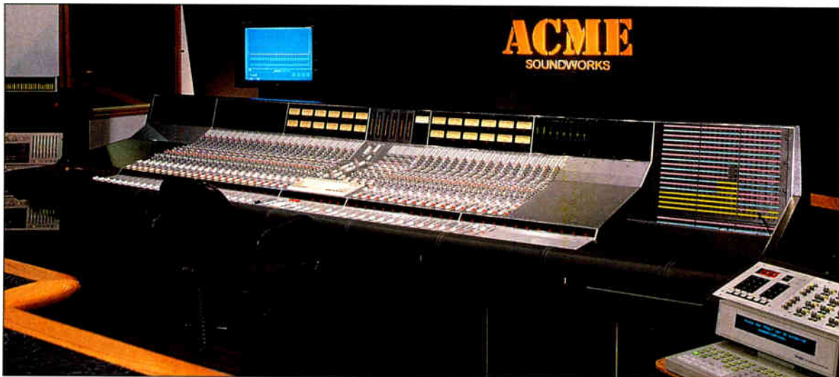
Lafont Chroma installed in Studio A at Acme Soundworks, West Los Angeles
