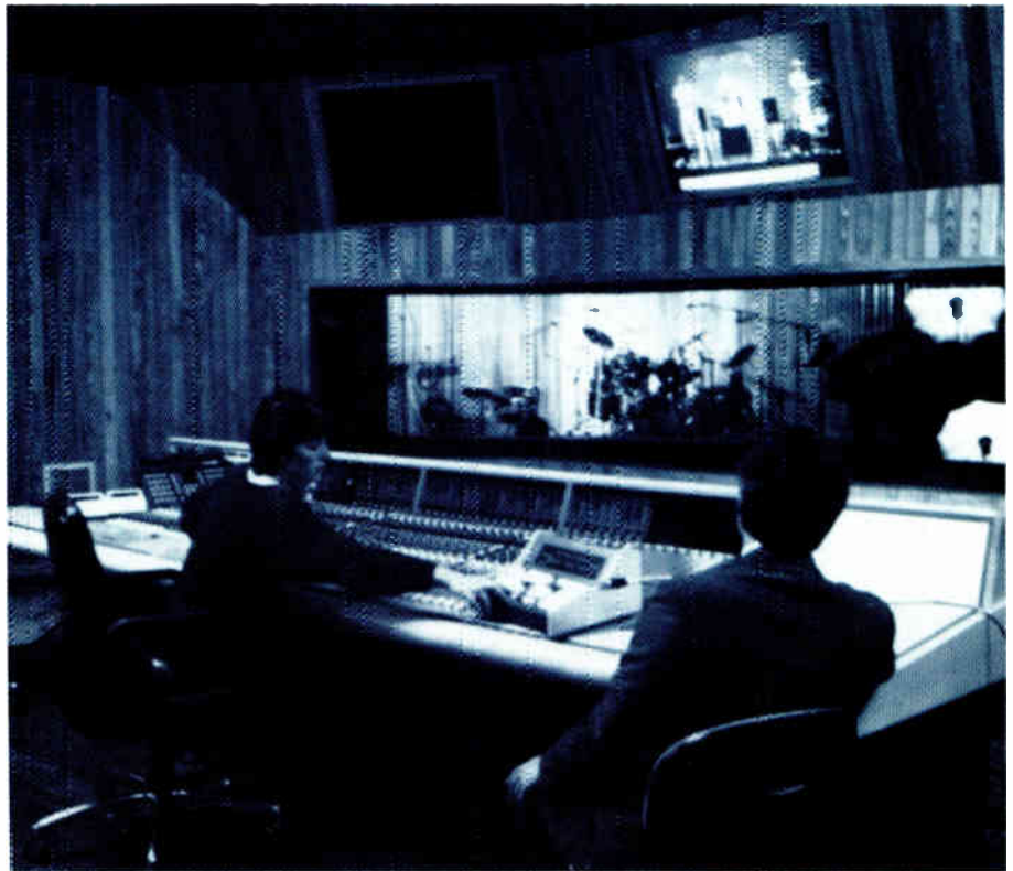
Crawford Post Production in Atlanta uses a Neve automated console with Studer tape machines to handle their audio-for-video needs.
