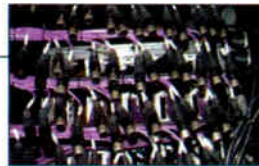
Neutrik connectors on Entravision's master control satellite-uplink audio distribution amplifier
