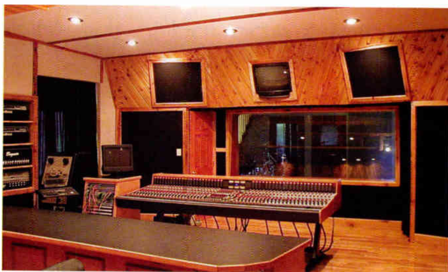
Cedar Rock Studios (Shelburn, Ind.) installed a Trident Series 80 5.1 console.
